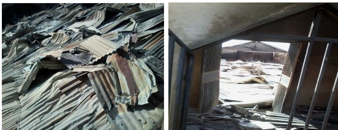
Burnt roofing sheets of one of the Evangelical Reformed Church of Christ at Yelwan-Bassa, Kokona LGA of Nasarawa state (Source: NCSAN)
